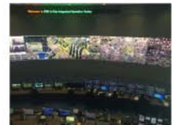
City Operation Center
