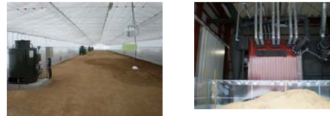
Wood biomass boiler at a seedling greenhouse
