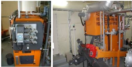
Wood biomass boiler
