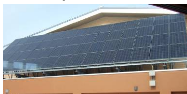
Solar panels on an elementary school
