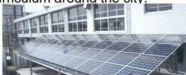
Solar power generation at Sone Higashi Elementary School
